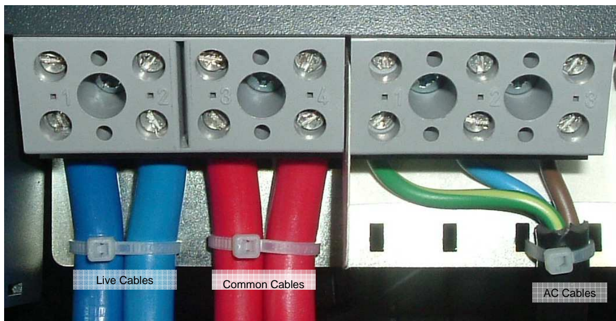
Fig 3. AC and DC cable strain relief
